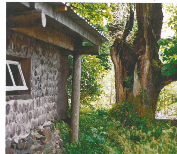
Hut sites work best with natural character retained as much as possible. Photo: Karen Grant
