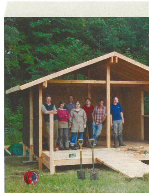
Participants on a timber frame building course with architect Duncan Roberts. Photo: Falkland Centre for Stewardship.
